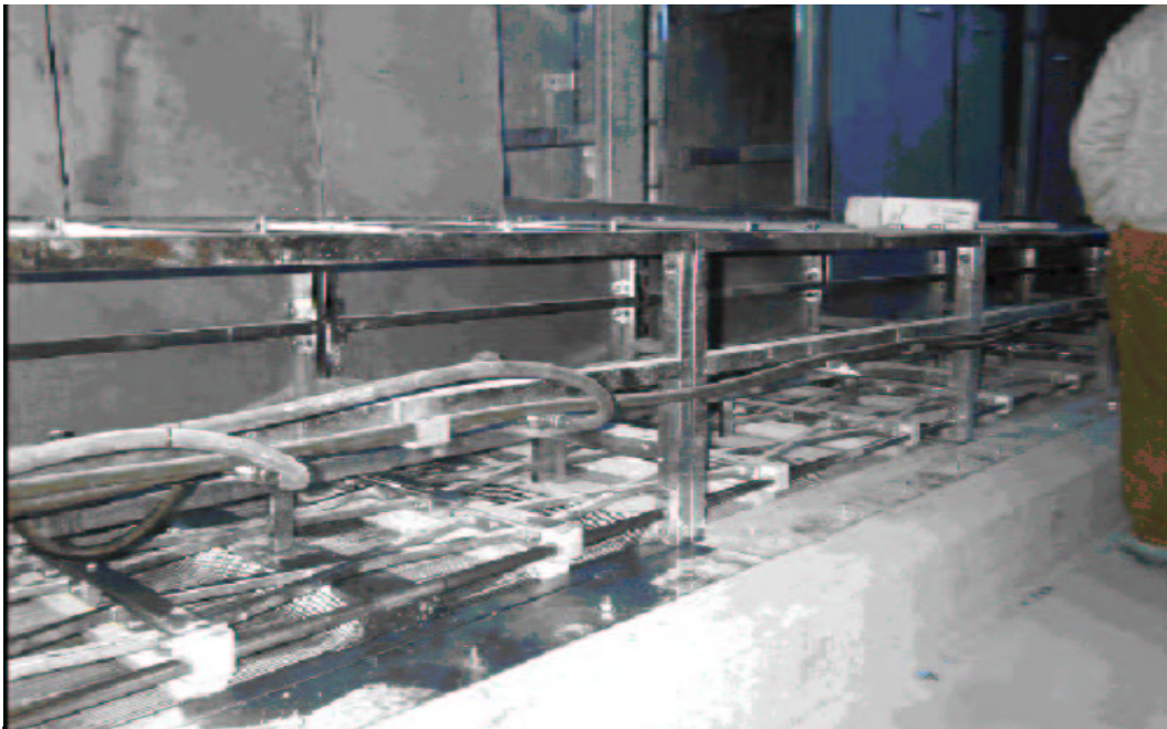
Horizontal bar racks at the Teall Brook Floatables Control Facility
