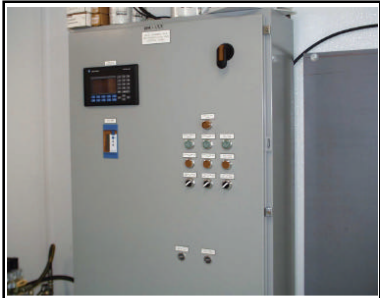
Erie Boulevard Storage System, Control Panel
