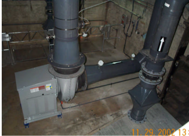
Picture 11 – New odor control system fan at Baldwinsville/Seneca Knolls WWTP
