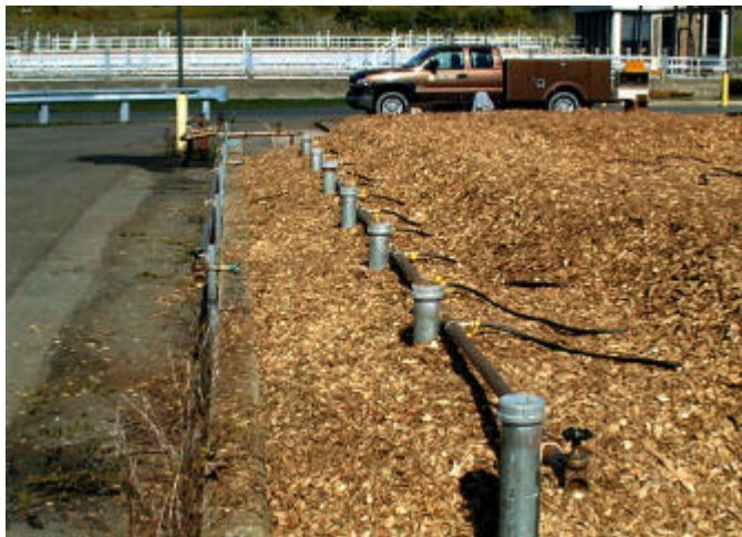
Picture 12 – New odor control system media bed for Baldwinsville/Seneca Knolls WWTP
