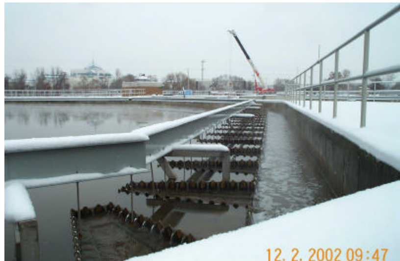
Picture 9 – New weir leveling system for secondary clarifiers at Metro WWTP
