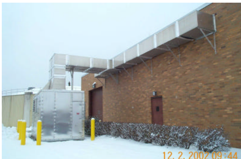
Picture 6 – New HVAC unit for Metro WWTP – Plant Maintenance Building
