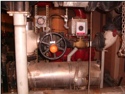
Hot Water Heat Exchanger
