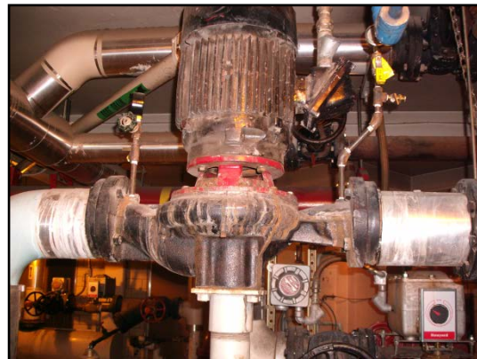
Hot Water Recirculation Pumps
