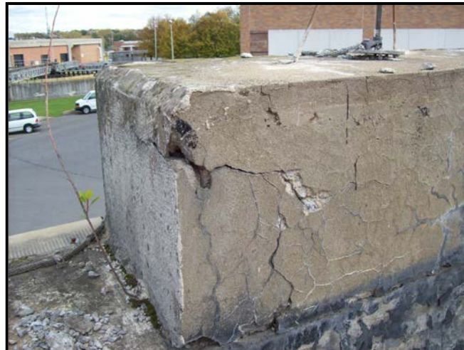
Photo 3: Pilaster Cracks and Vegetative Growth
