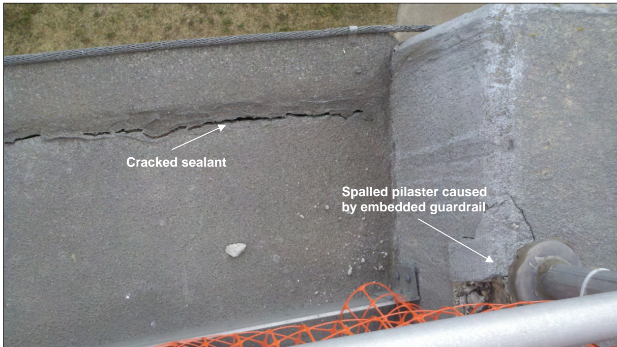
Photo 1: Top of Digester No. 1 exterior wall, looking down on parapet extension and sealant along metal siding flashing cap.
