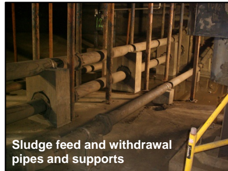
Sludge feed and withdrawal pipes
